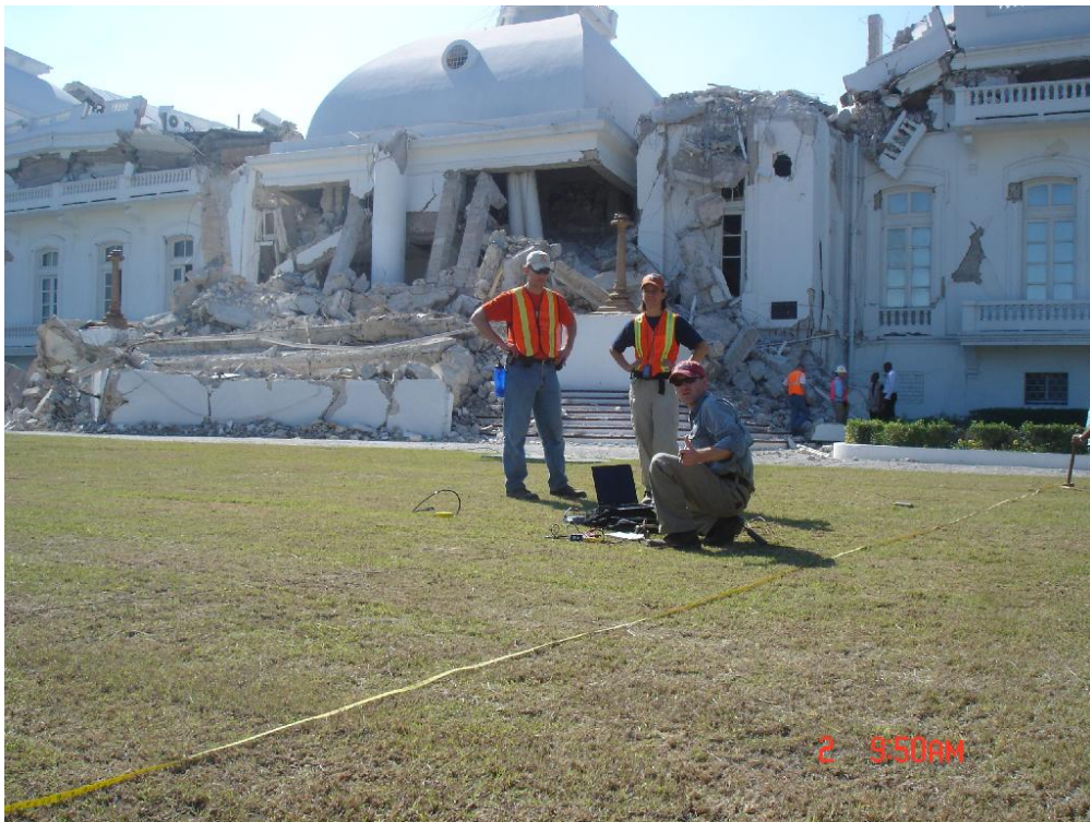
Figure 5.9 The Presidential Palace lies within the heavily damaged zone noted above. Two SASW tests and one H/V Spectral Ratio test were conducted here (N 18.543633°, W - 72.338905°).
